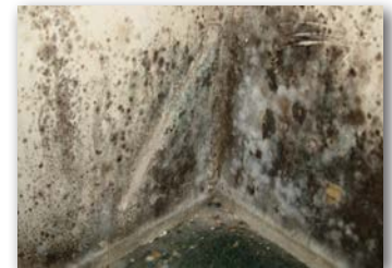
Water Damage & Mold in Wood Home
